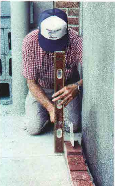
Maintaining plumb and level. Check the first brick for vertical alignment with the modular scale rule (top), then level its top (middle photo) and plumb its face (above). Repeating this procedure at the opposite end of the wall gives two points to pull a line from.
