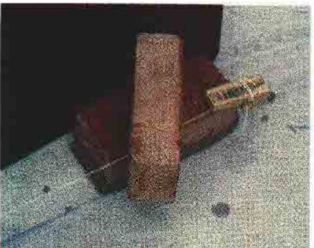
A line block hooked over one end of the wall is held in position by a line block at the other end. A dry brick set on top of the line sets it in the plane of the face of the wall.
